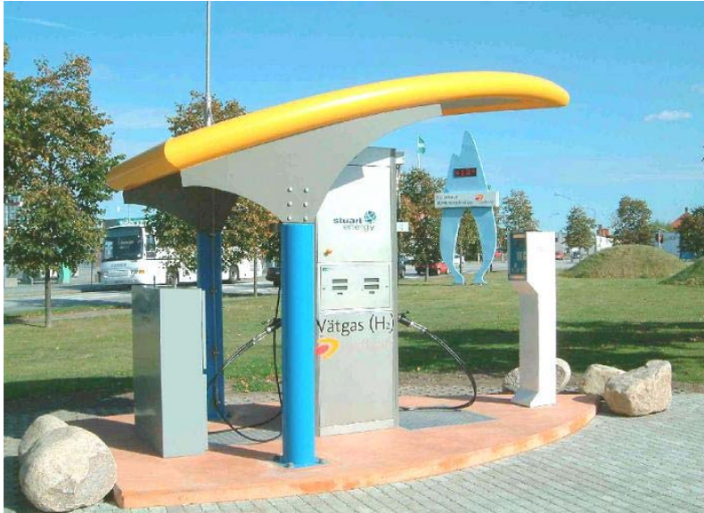
Fig 3. Dispenser hydrogen and mix of CNG/hydrogen
