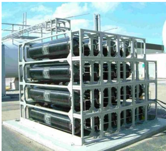
Fig 1. Hydrogen storage pressure tanks
