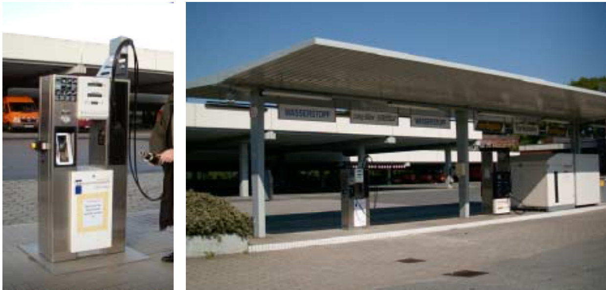
Figure 8: Hydrogen dispenser and filling station
